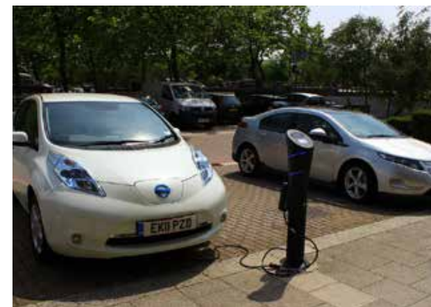
Electric car charging points
